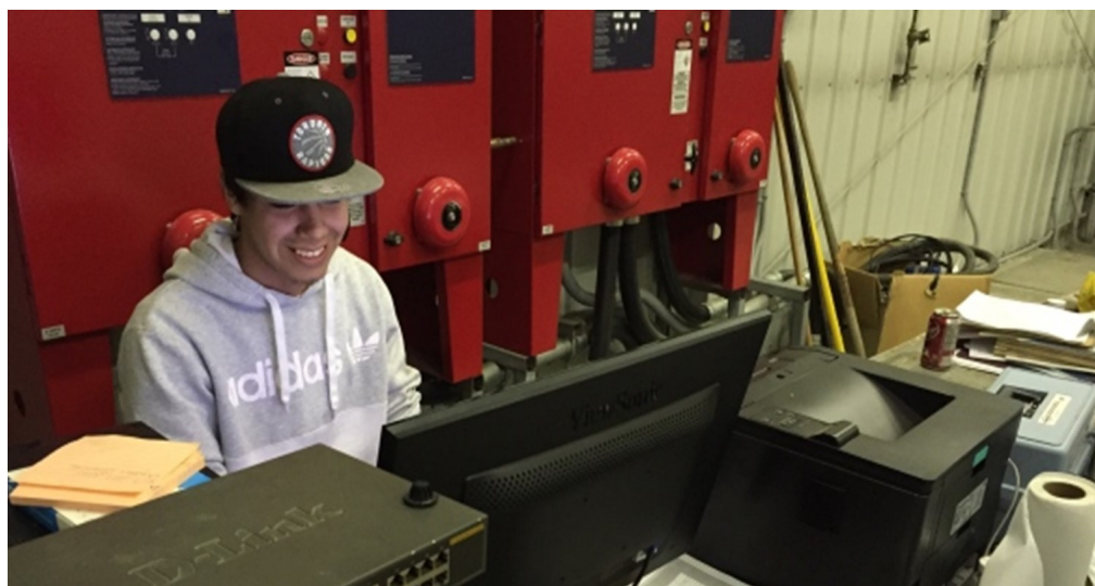
Quentin Rae, 19, files the water monitoring reports at the North Spirit Lake First Nation water plant.
